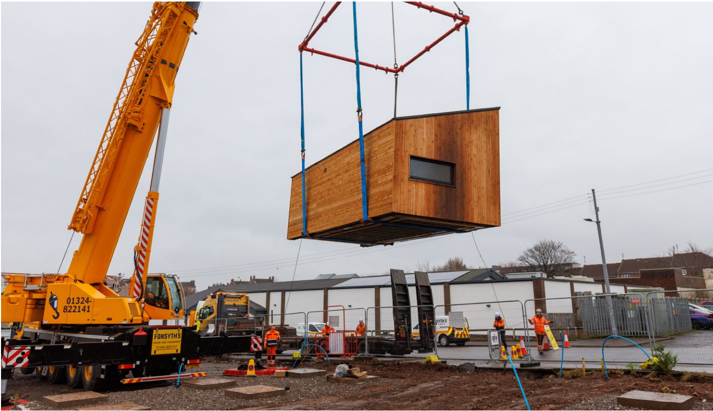
A house arriving on site at the Social Bite Village in Rutherglen, South Lanarkshire
